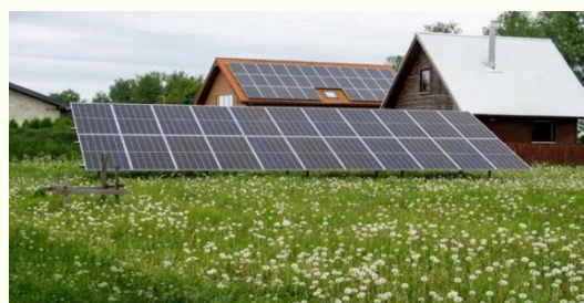
Figure 7 Ground mounted solar from EnergyHub
