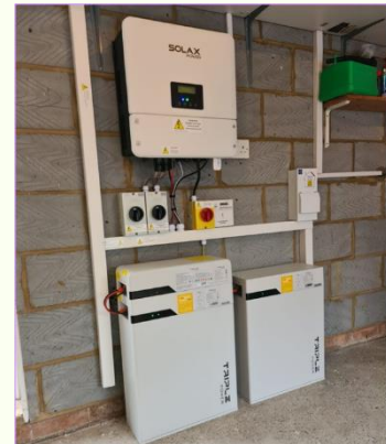
Figure 4 Solar battery storage from TheSolarShed.co.uk
