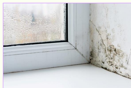
Figure 1: Window condensation and subsequent mould growth. Source: Pure Earth Collection
