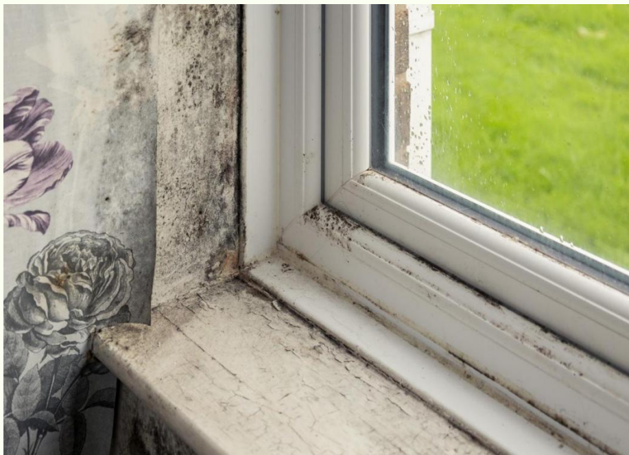
Figure 1: An example of mould within the home. Source: West Lindsey District Council
